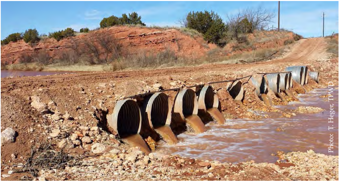
Figure 23 - Culverted crossing removed from the Double Mountain Fork Brazos River located in the Upper Brazos River Native Fish Conservation Area.
