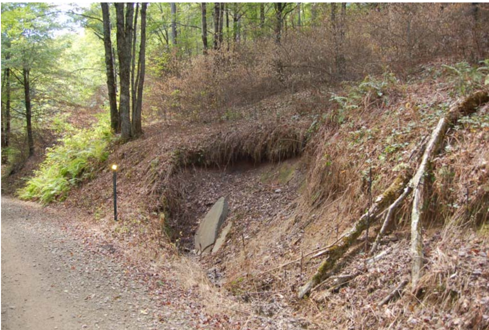
Improper drainage from unimproved dirt and gravel road adjacent to Class A native brook trout stream. Photo by Amy G. Wolfe, Trout Unlimited
