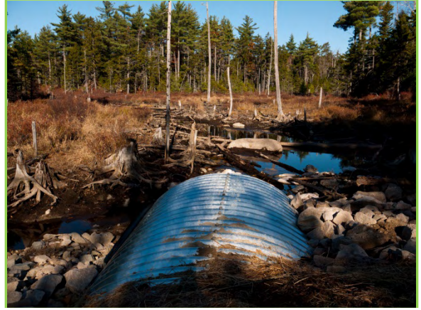
Figure 13: Black Rock Brook downstream following installation of new culvert. Photo by Nancy Sferra.
