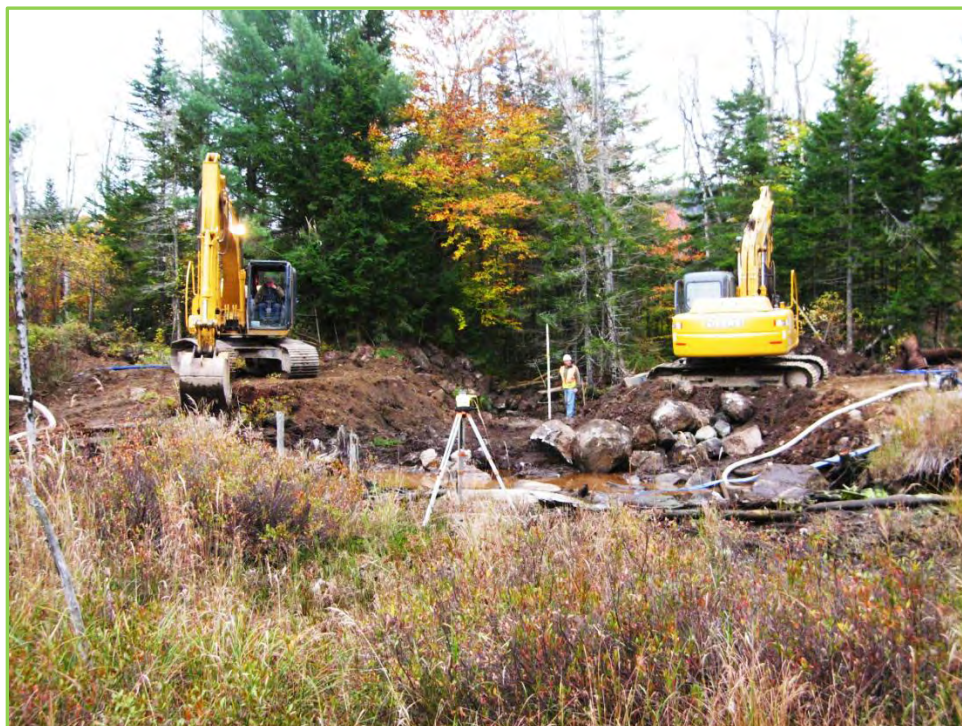
Figure 5: Construction work at Black Rock Brook site, October 2011. Photo by Dan Grenier.
