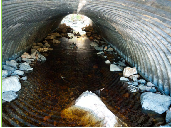
Figure 15: Black Rock Brook culvert looking from the upstream side. Photo by Nancy Sferra.
