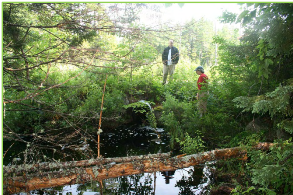
Figure 12: Black Rock Brook upstream of culvert before restoration. Photo by Scott Craig.
