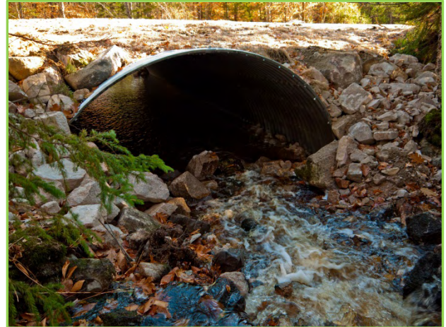
Figure 10: Ash Bog Stream upstream of culvert following installation of new culvert. Photo by Nancy Sferra.
