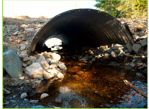
Figure 16: Black Rock Brook culvert looking from the downstream side. Photo by Nancy Sferra.
