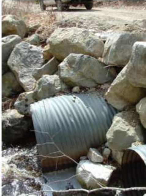
Photo 1: Outlet of culverts at Ash Bog Stream. Outlets are perched during most of summer and undersized culvert leads to overwash and sedimentation into the stream. (Photographer: Nancy Sferra, The Nature Conservancy).
