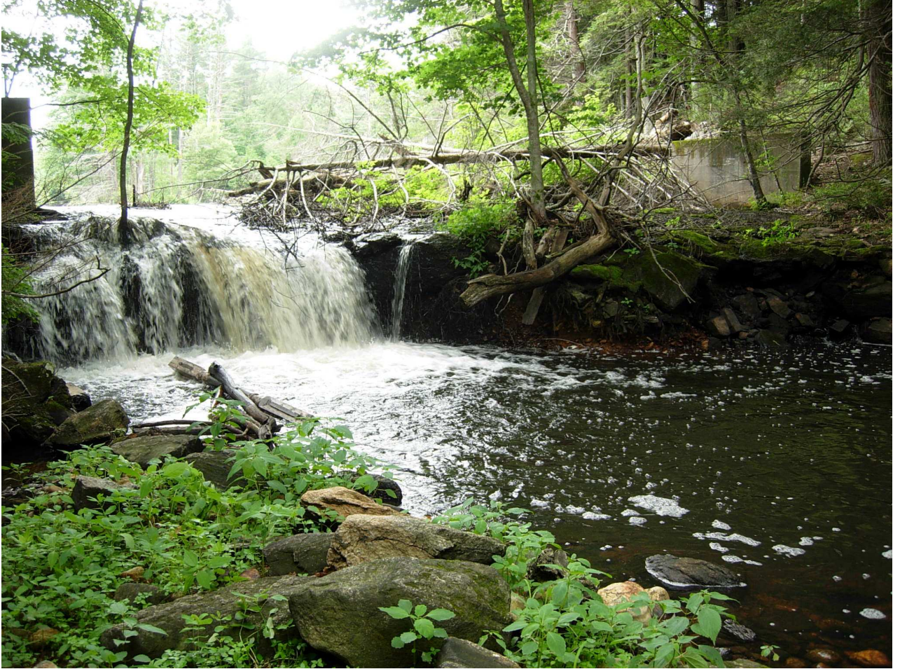
Failing dam on upper impoundment. A.Norris, MDFW.
