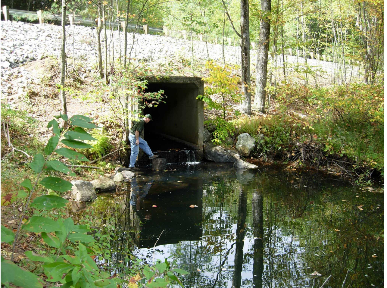
Perched, undersized culvert at mouth of Hamant Brook. A. Norris, MDFW
