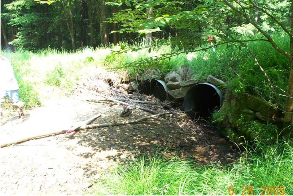
Figure 2: Inlet (upstream) for culvert 116/2. Note the accumulation of debris and near complete closure of the culvert on the far left. Photo courtesy of Brent Pence (USFS).
