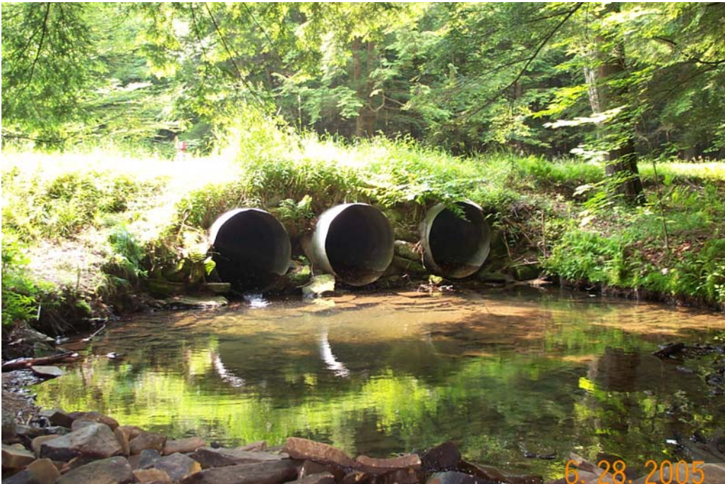
Figure 3: Outlet (downstream) for culvert 116/2. Note the elevation between the culvert ends and the water level, and the concentration of flow through only one of the three culverts. Photo courtesy of Brent Pence (USFS).
