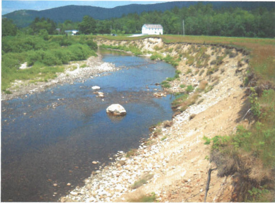
July 6, 2010, Bear River Grange, prior to construction. View upstream. Photograph by Jeff Stern, Androscoggin River Watershed Council.
