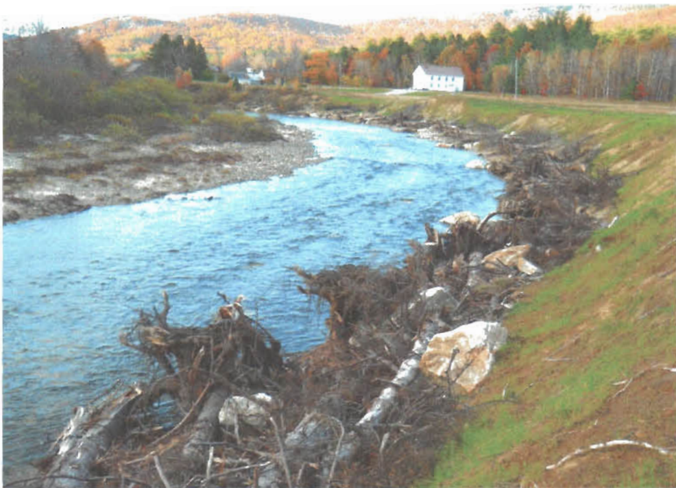
October 18, 2010, Bear River Grange, after construction. Photograph by Jeff Stern, Androscoggin River Watershed Council.
