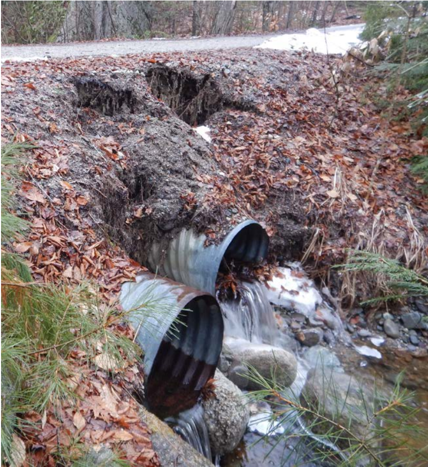
1: Before: culvert outlet w/ erosion after fall storm
