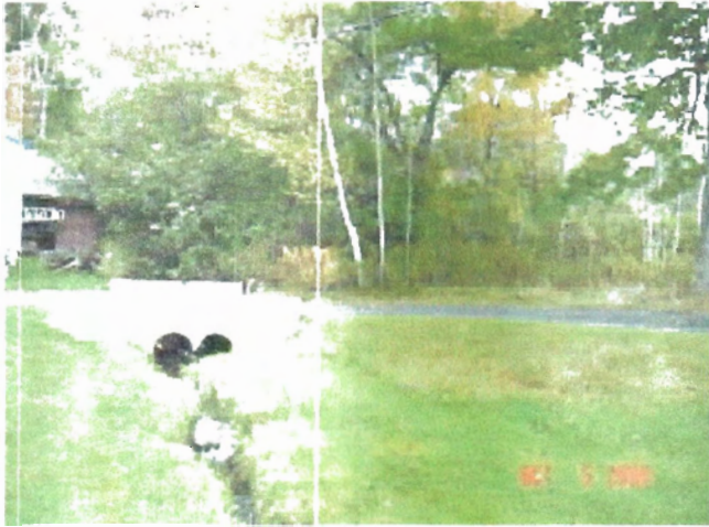
Belfast, Maine: Unnamed Stream, existing culverts (upstream of dam). Photograph: W.L. Woodward, Oct. 5, 2006
