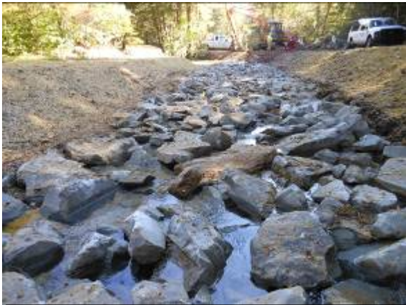
Photo 7 – Completed infiltration gallery. Note flow through interstitial spaces. Through time these should fill in with natural bed material. credit: PFBC
