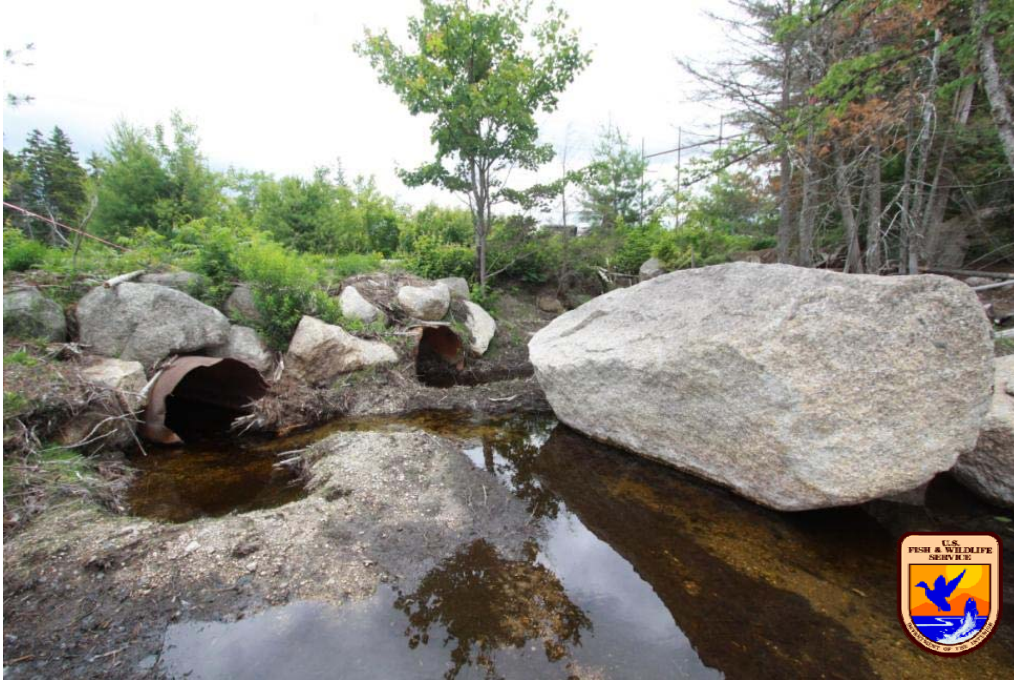
Looking downstream to old culverts at the outlet stream to Knox Lake (n=2 culverts).
