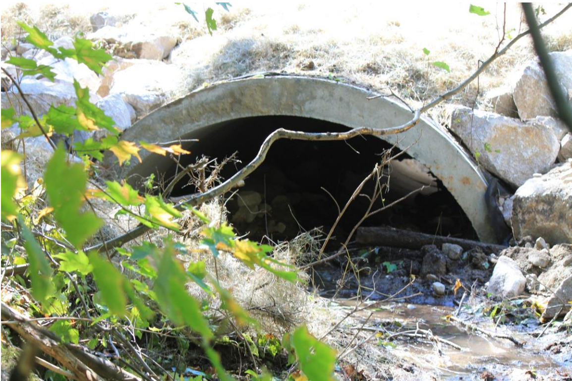
Billy Brown Brook at Shaw Street crossing after arch culvert installation in 2014.
