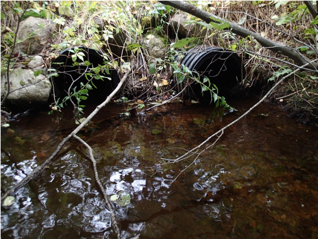
Billy Brown Brook at Shaw Street crossing prior to arch culvert installation in 2014.
