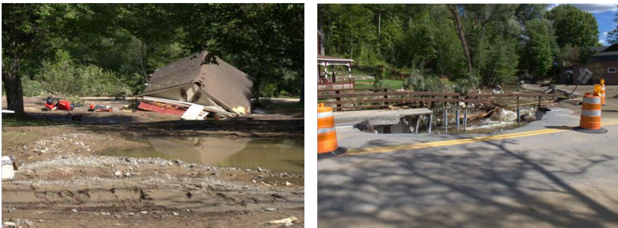
Figure 1: Tropical Storm Irene Damage in the Ausable River Watershed
