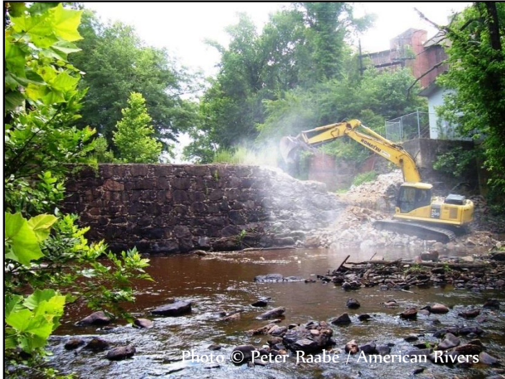
Figure 4-3: Steeles Mill Dam on Hitchcock Creek in North Carolina during and after removal in 2009
